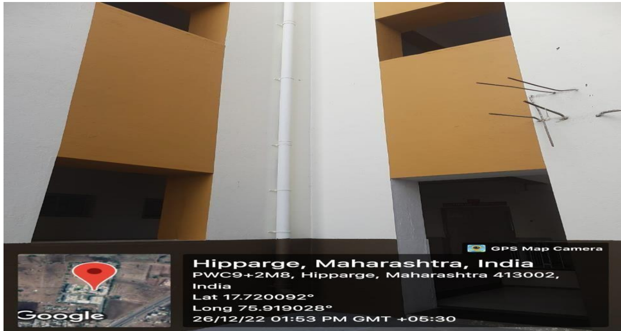
Figure 48: Pipes attached to the roofs of the buildings
