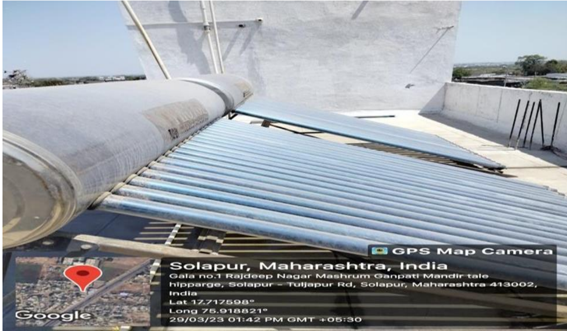
Fig 17: Solar Water Heater installed in Boys Hostel's top floor which helps in reducing electricity consumption
