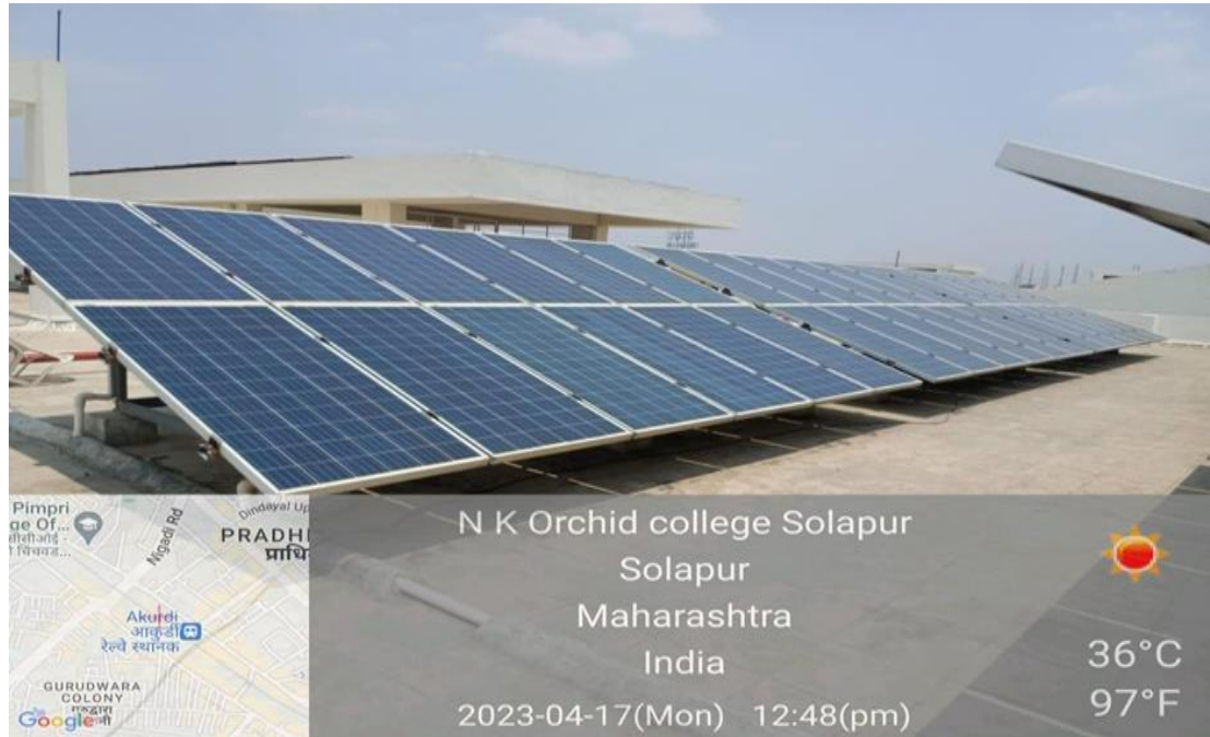
Figure 1: 36 KW Solar Power Generation System
