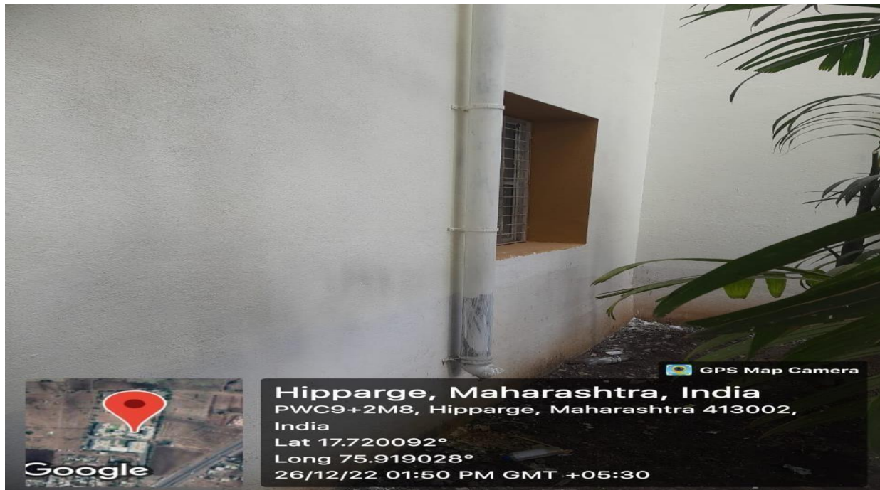
Figure 49: Pipes attached to the roofs of the buildings
